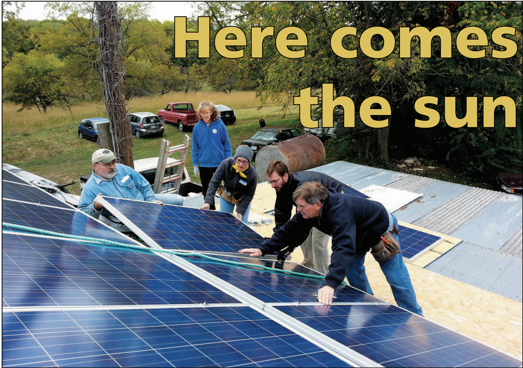
From left Jim Sherow, Madonna Stallmann, Cherri Harper, Ben Champion and Mike Life install solar panels at Cherri Harper and Jacque Gibbons' home at 10520 Harvest Road between Manhattan and Wamego. Photos courtesy Cherri Harper
